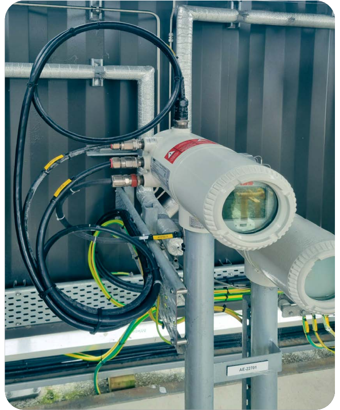
Figure D6. GC at Te Horo DP.
