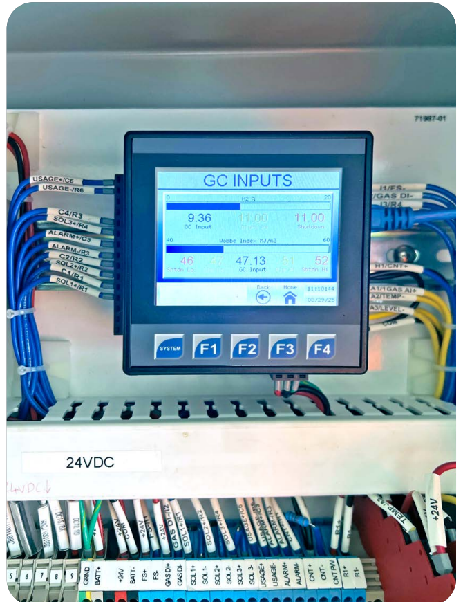
Figure D9. Welker PLC at 10% stage.
