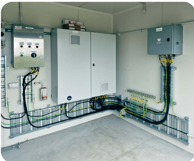
Figure D3. Solar & PLC container at the DP.
