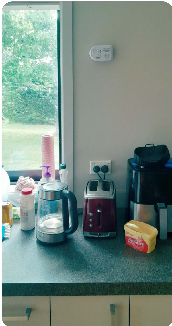
Figure 16. CO Monitor installed at property #5.
