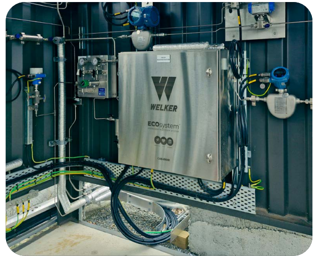
Figure 1. Welker unit set up at the DP
