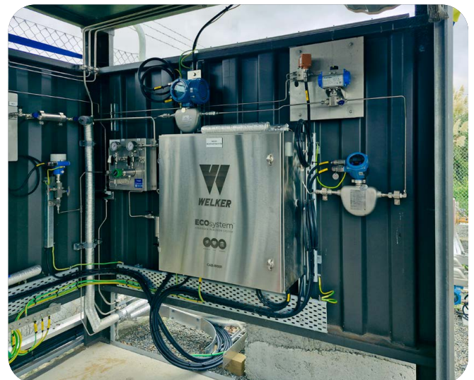
Figure D4. Welker H 2 injection & GC container at the DP.
