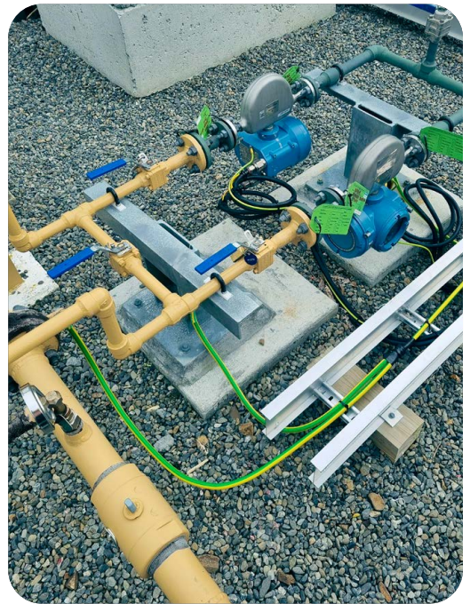
Figure D2. Gas meters piping at the DP.
