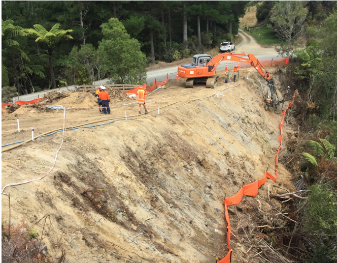
Figure 11: 400 line erosion remediation at Awakau
